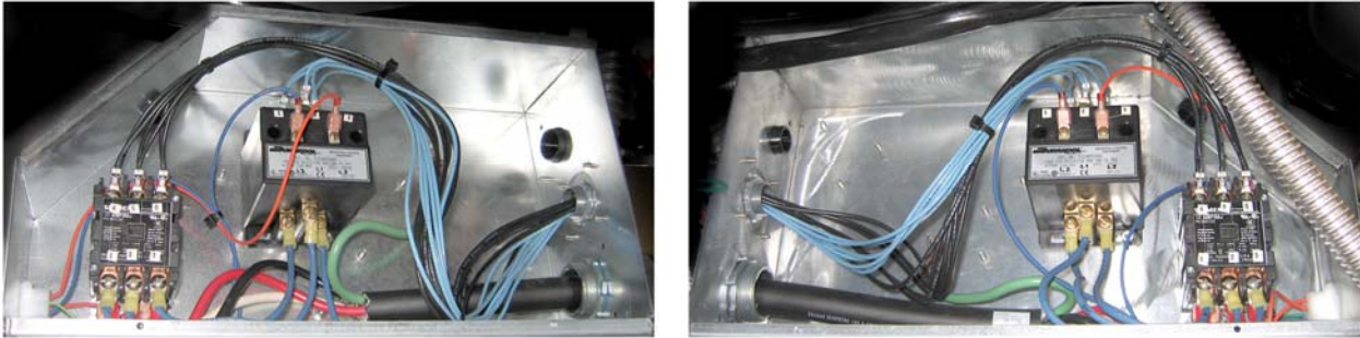
Left and right views of mechanical contactor box components.
